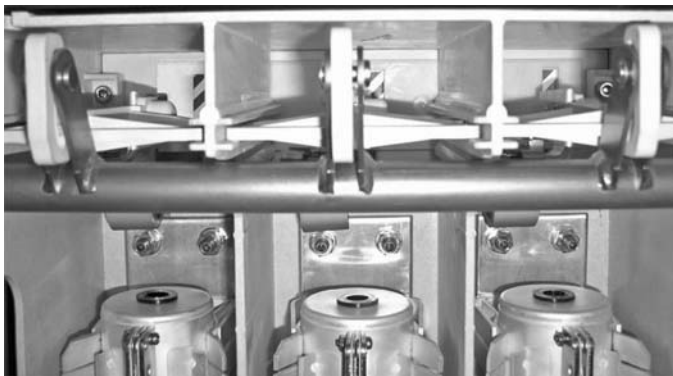
View of Isolation Switch Through Viewing Window
