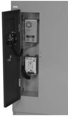
Lower Compartment Low Voltage Door
